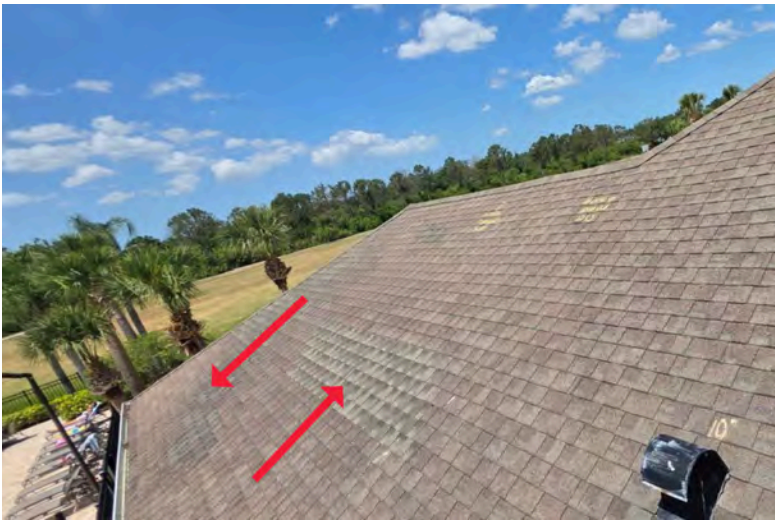
Previous repair areas
