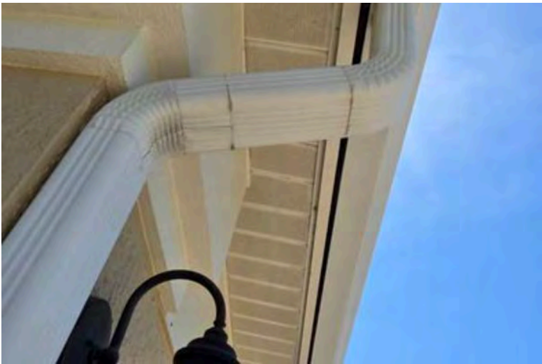
Adequate intake ventilation: perforated soffits
